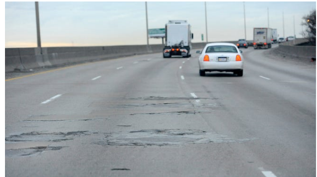
Figure 5 – Deck Conditions Prior to Project
