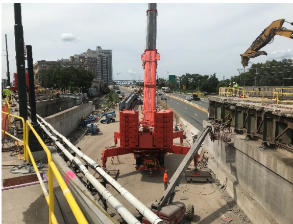
Photo 16 – 600 Ton Mobile Crane in I-90 during Outage 2 Setting New Girder Around Live KV Lines
