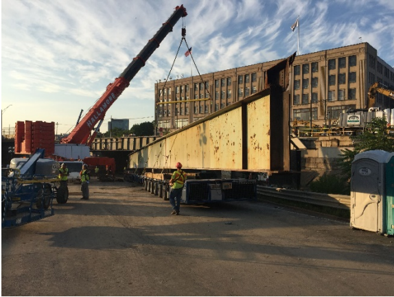
Photo 13 - SMPT Loaded with Girder during Outage 2 to be Transported to Processing Location
