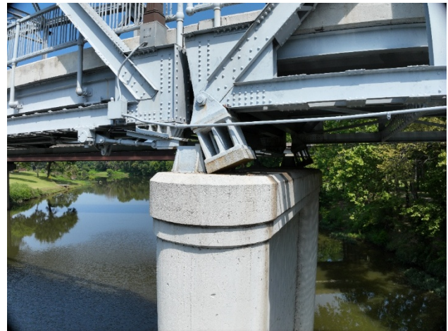
IMG 2 - Damaged Pier
