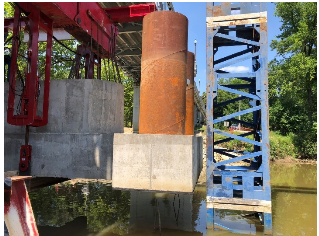
IMG 6 - Tight Clearance
