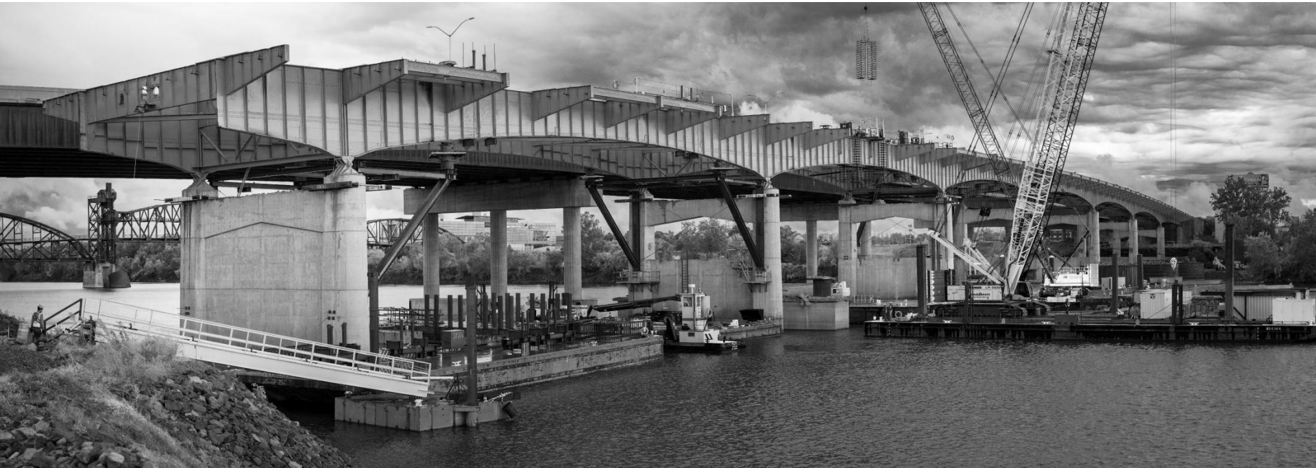
30 Crossing Construction. Panorama demolition old I-30 bridge at Pier 24, North Little Rock, Arkansas. October 25, 2022. ©David Hoge IMM03195-pano.ar
