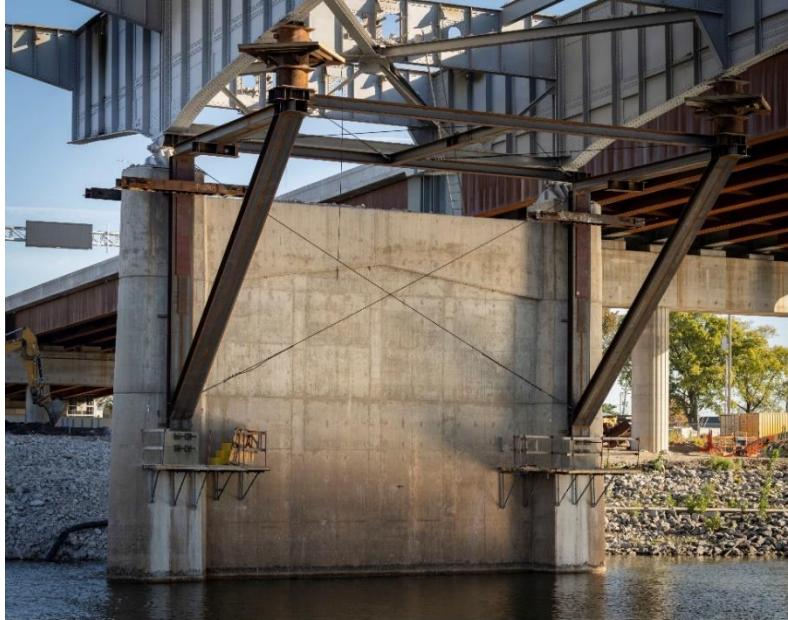
30 Crossing Construction Pier 24 with pier brackets. Demolition of I-30 bridge, North Little Rock, Arkansas, October 20, 2022. ©David Hogg
