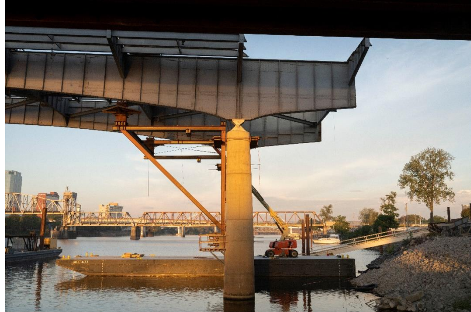
30 Crossing Construction Pier bracket on P-21. Demolition of I-30 bridge, North Little Rock, Arkansas, October 12, 2022. ©David Hogg
