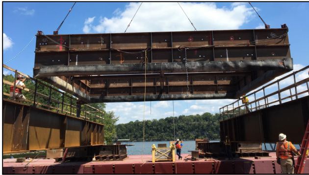
Photo 5 – Steel frame used to form the tremie concrete above the bottom of the lake
