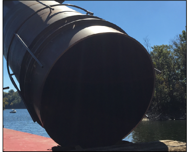
Photo 6 - Radial Bearing PL Added to Permanent Casing for Shear Load Transfer to Tremie Concrete
