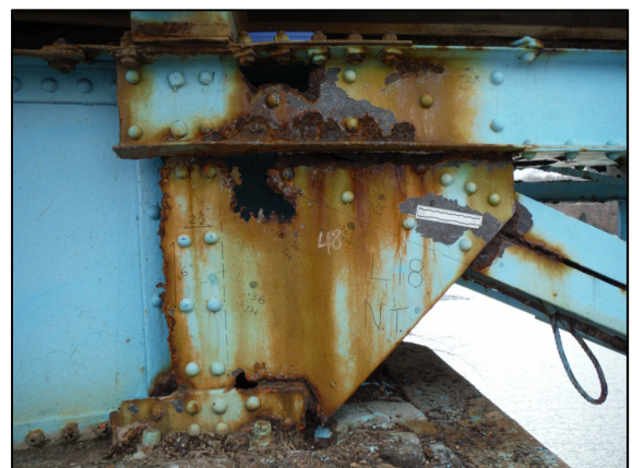
Photo 2 – Existing Truss in Poor Condition
